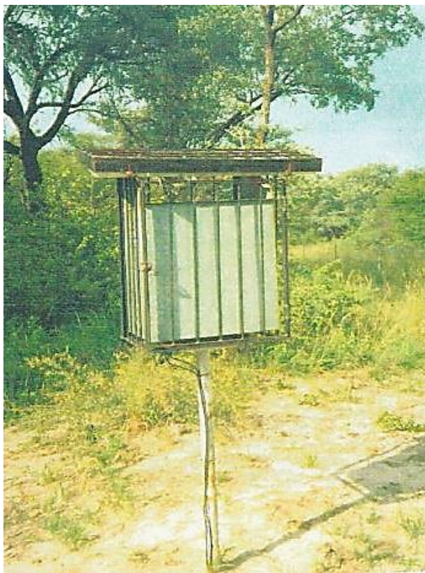
Plate 7: An example of a protection box from which solar panels and energisers have been stolen
